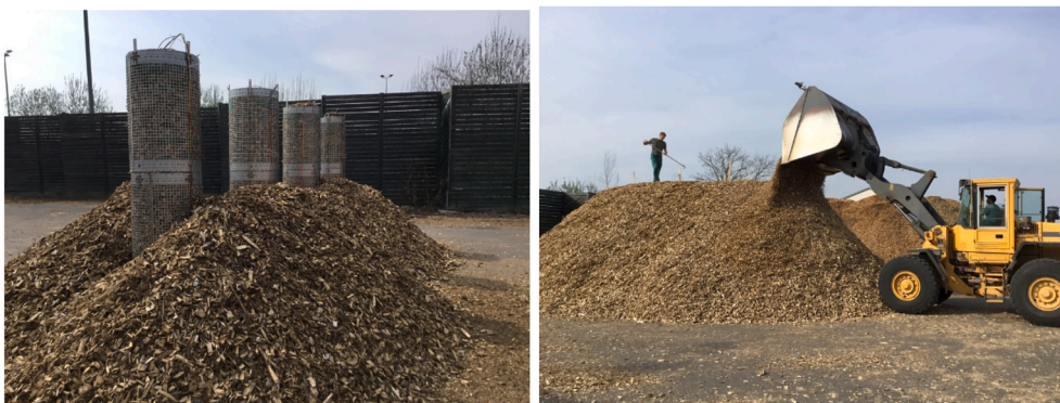
Fig. 1. Installation of the measuring columns (left) and construction of the wood chip piles (right).
